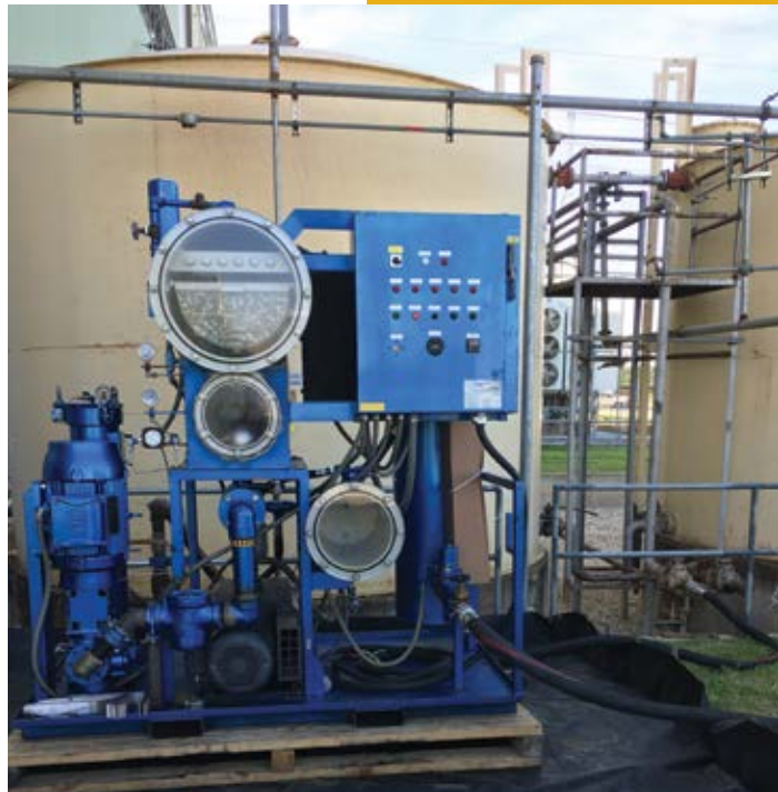
50 GPM VDOPS rental unit at a power plant in Texas
